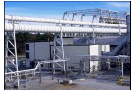
Arnold Air Force Base 320,000 cfm Low-Pressure Refrigerated/Desiccant Air Dryer
