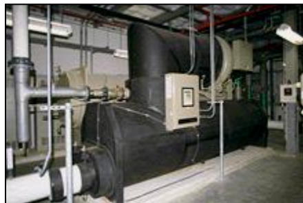
1,000 hp Glycol Chiller at Client's Site
